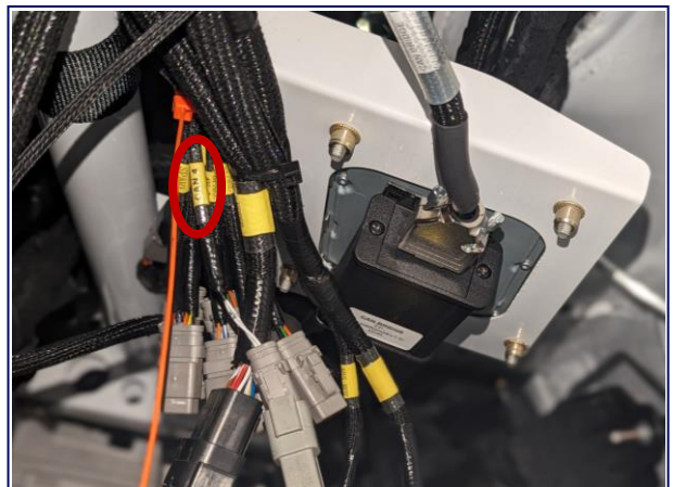
VBOX Wiring Labeled "CAN4" Underneath Dash
