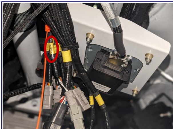
VBOX Wiring Labeled "CAN4" Underneath Dash
